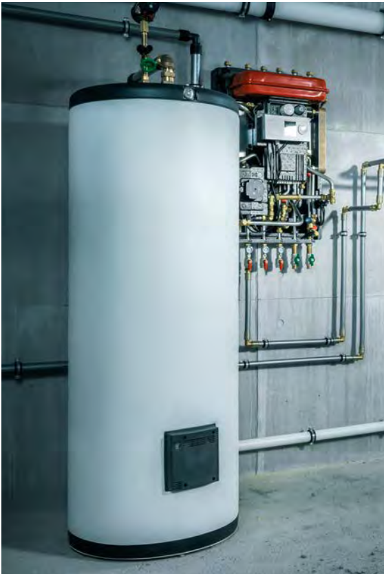
Fig. 06-9 Decentralised heat store
