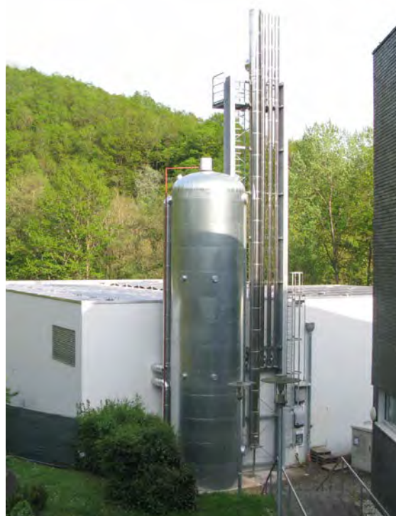
Fig. 06-8 Central heat store
